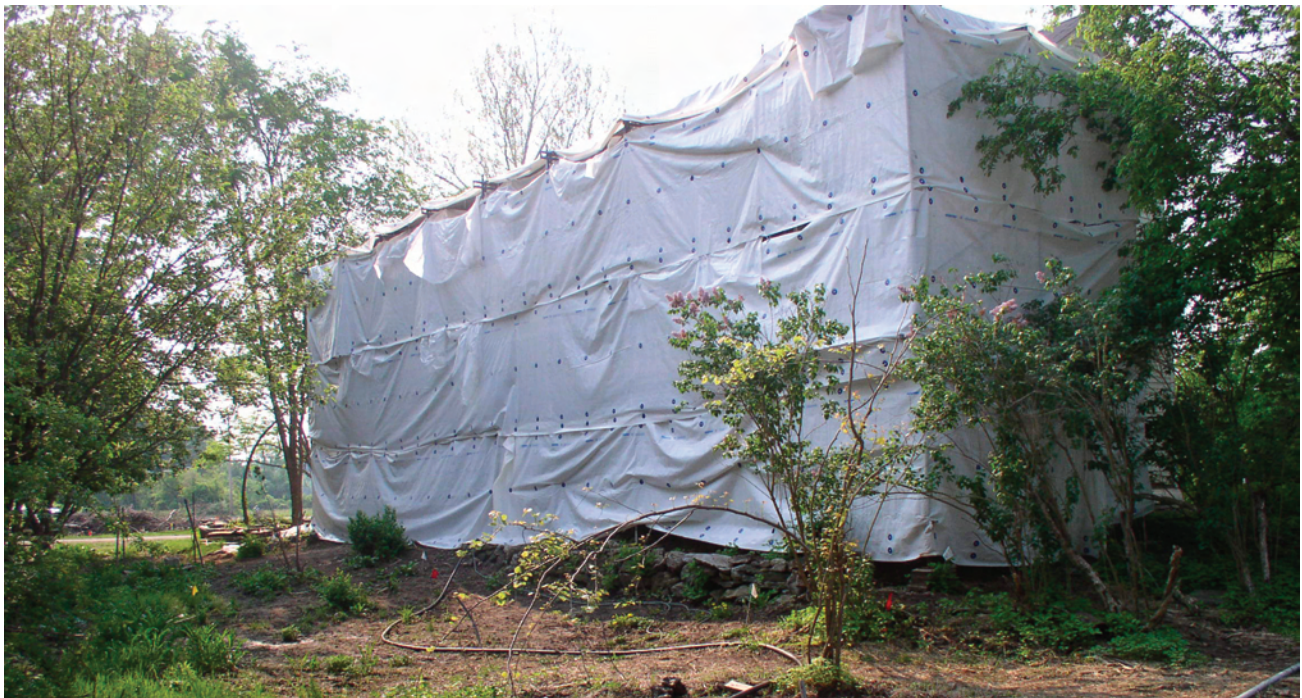
Figure 4. View of the scaffolding covering the north face of the house in 2007.
